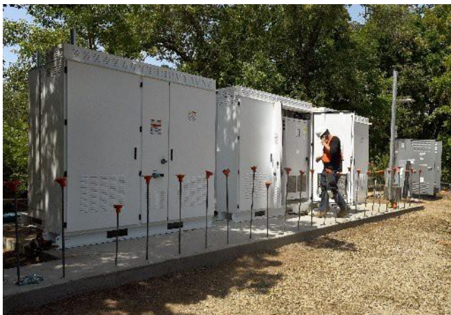
Figure 4: Energy Storage Installation at College of Marin
