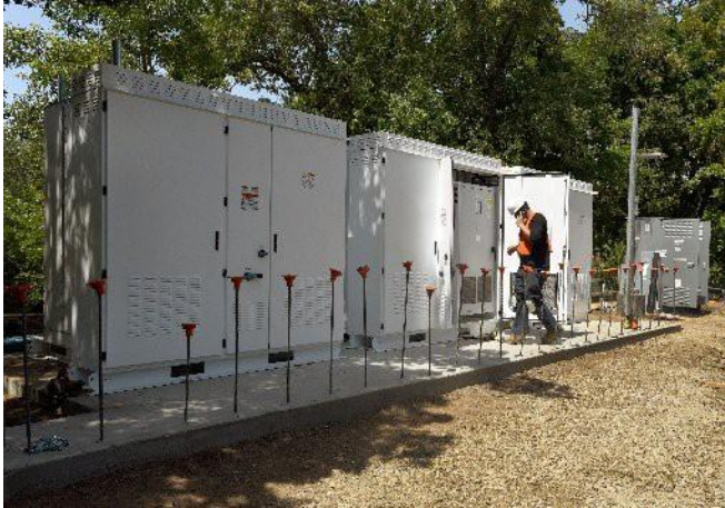
Figure 4: Energy Storage Installation at College of Marin
