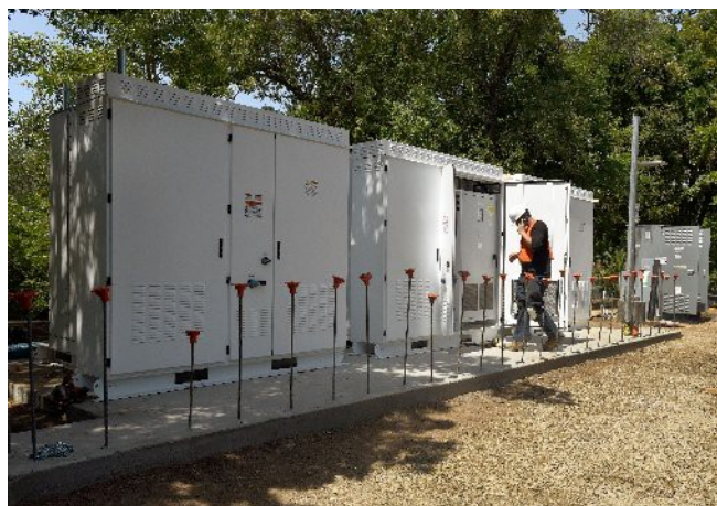
Figure 5: Energy Storage Installation at College of Marin
