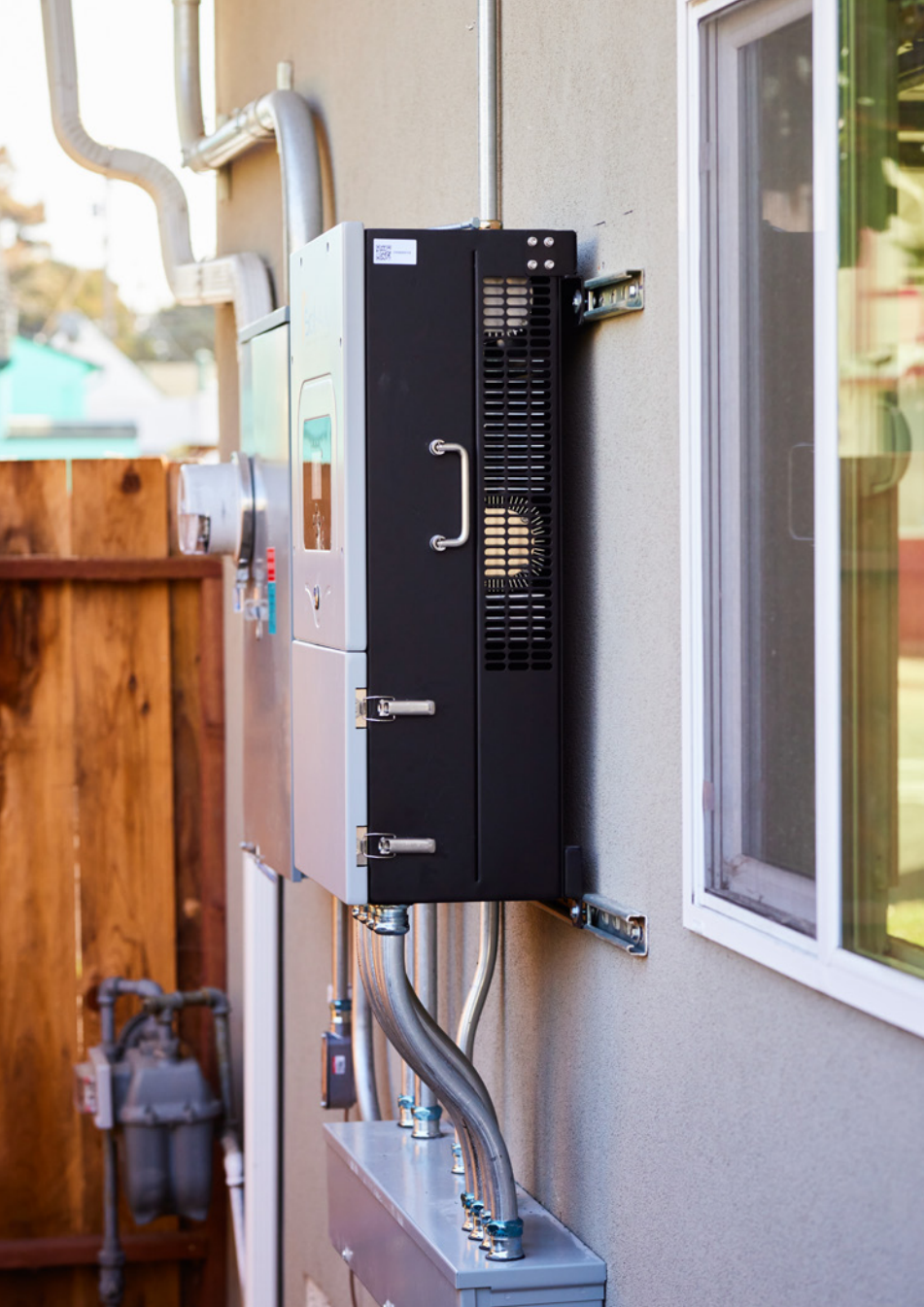
Electrification equipment connected to MCE's Richmond VPP Pilot.
