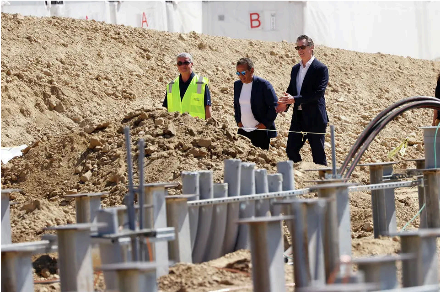
FILE: California Gov. Gavin Newsom, right, former Mayor Antonio Villaraigosa, center, and Jim Shandalov, vice president at NextEra Energy Resources, walk along the construction of the battery energy storage systems for the future site of Proxima Solar Farm on May 19, 2023, in Stanislaus County, Calif.
