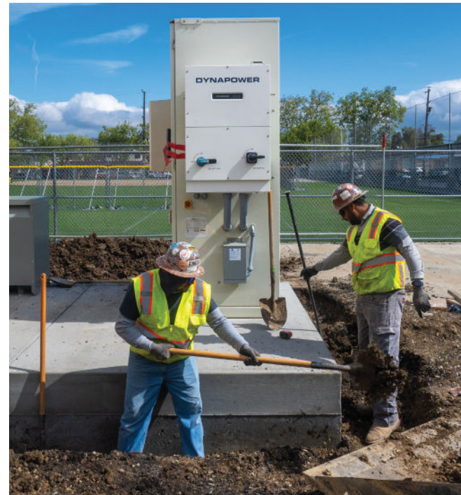
◀ A battery is installed at the Pittsburg Unified School District through MCE's Energy Storage program.
