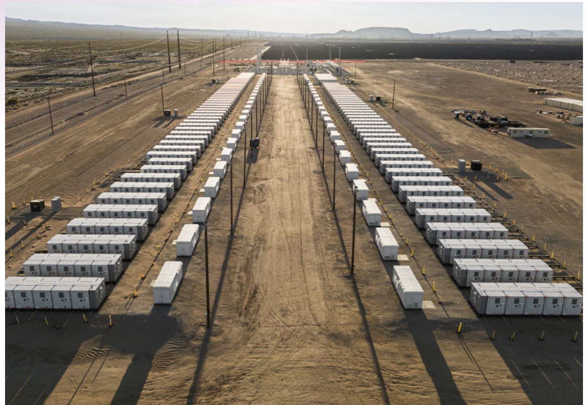
▲ Clearway’s Daggett Solar-Plus-Storage project in San Bernardino County supplies electricity to more than 181,000 homes.
