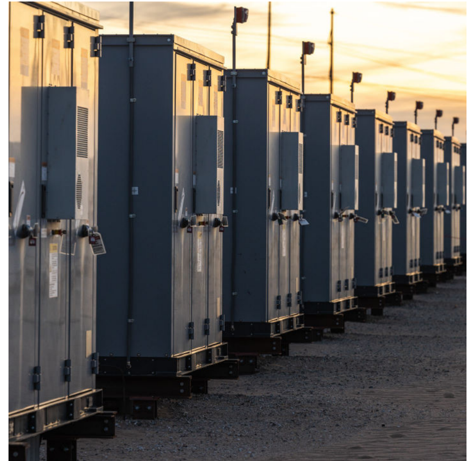
Daggett Solar + Storage Project
